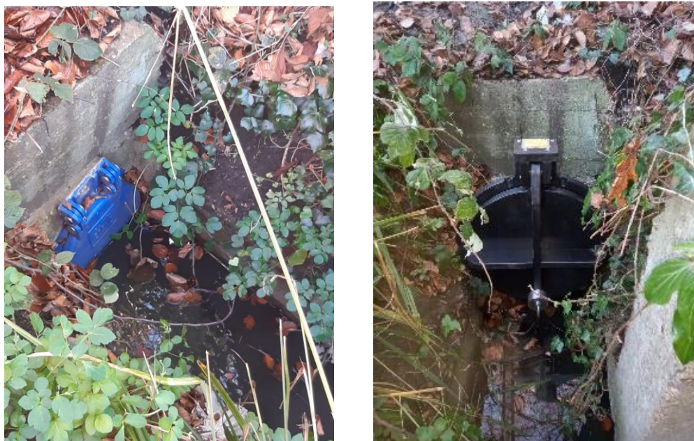
Figure 16 – Flap valve to ditch: Blue original (cast iron) black new (plastic)
