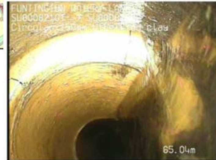
SU80082101Y_736de3af-8988-4446-ba3d-e880cc677ac4_20 240808_141000_206.jpg, 00:08:15, 65.04 m Infiltration, gushing at joint at 3 o'clock
