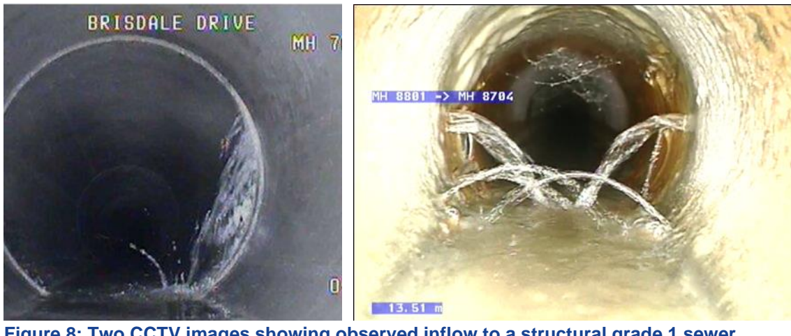
Figure 8: Two CCTV images showing observed inflow to a structural grade 1 sewer
